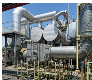
Solvent recovery equipment exterior
