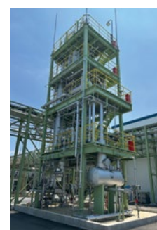
Solvent distillation equipment exterior
